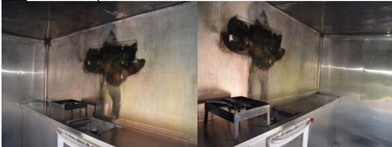
Demonstration/mock kitchen stove area (including the front of the stove)
